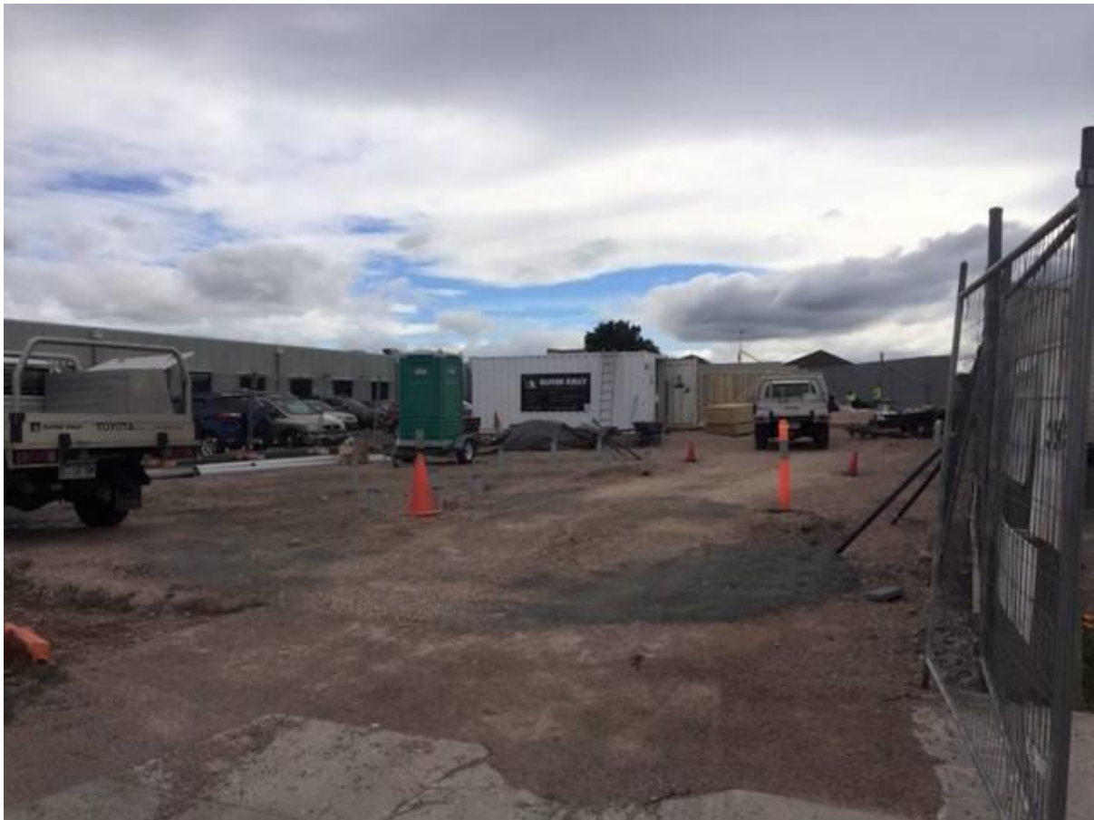
Housing Development: Work is underway on an 11 apartment social housing project in William Street in Devonport. Picture: Libby Bingham.
